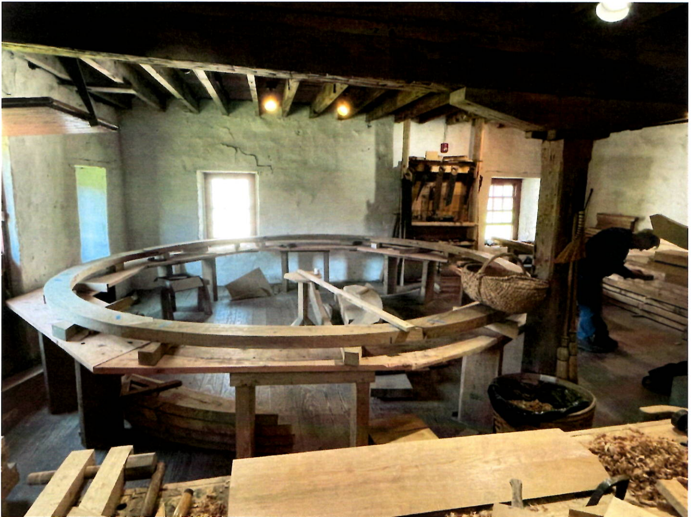
The millwright shop where staff and volunteers are fabricating the water wheel using 18 th century tools and techniques as an experimental archaeology project.
