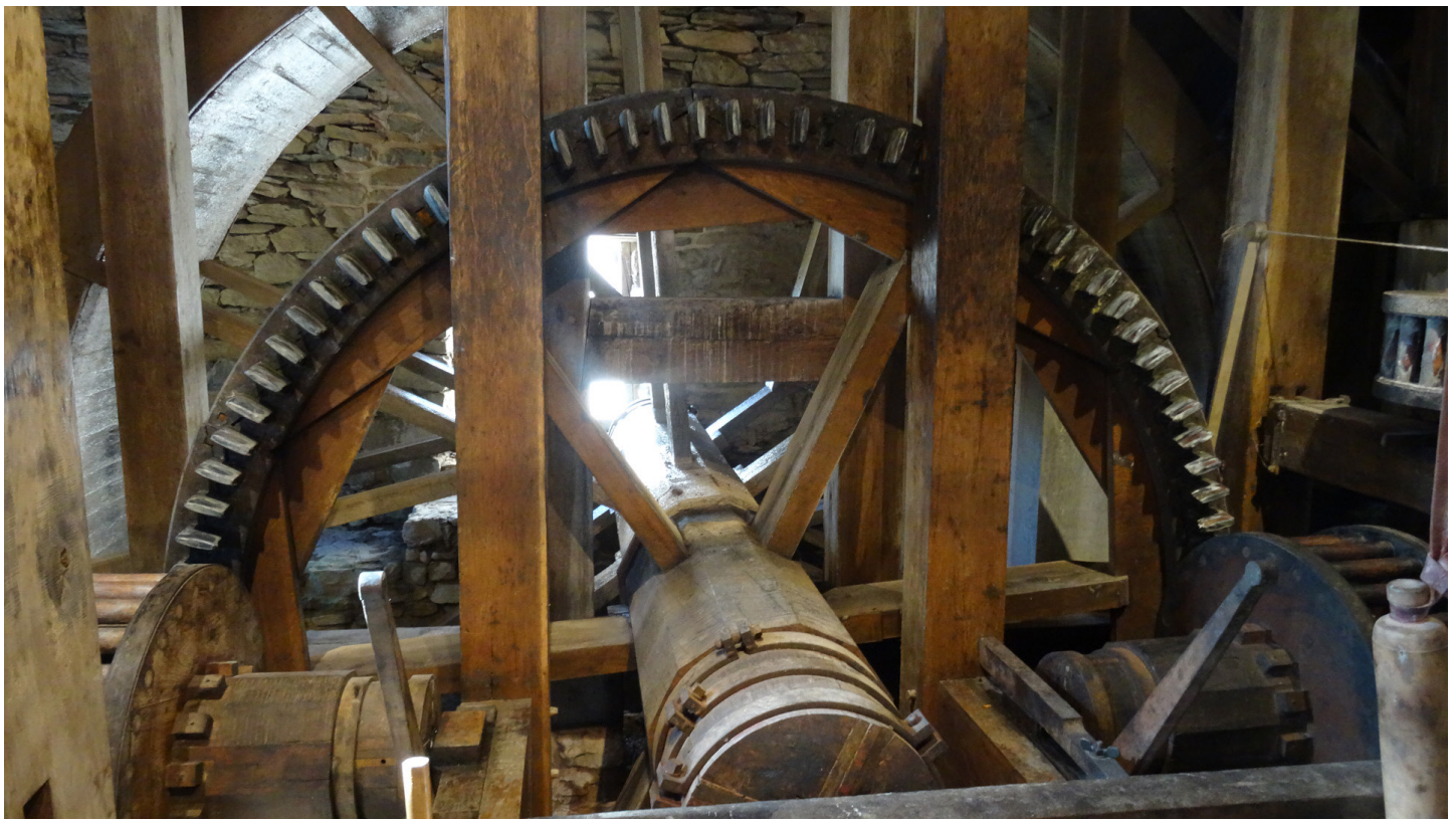
Burwell-Morgan Mill, showing the missing cog before being replaced (see cover photo).
